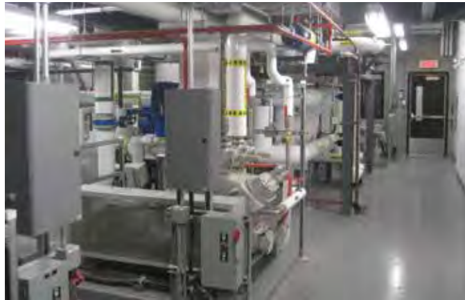
Mechanical room example – Michel-Normandin Arena, Montreal.
